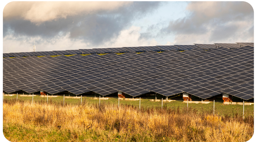
Photovoltaic power station Paracatú - MG
